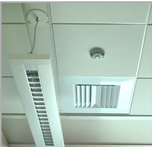
Occupancy Sensor Photo: Harvard Green Building Services
