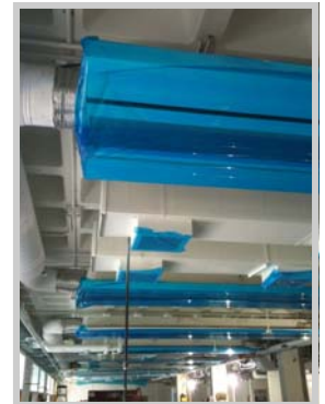
Sealed Ductwork Openings
